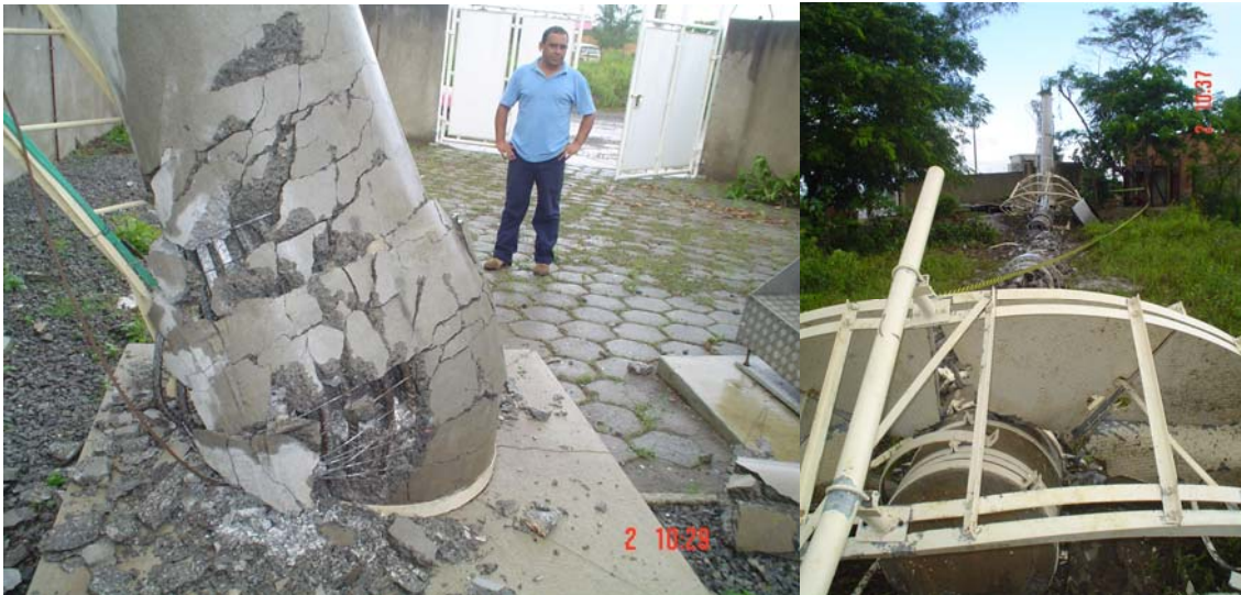
Fig. 2 – Pre-cast RC structure collapsed during a wind storm
