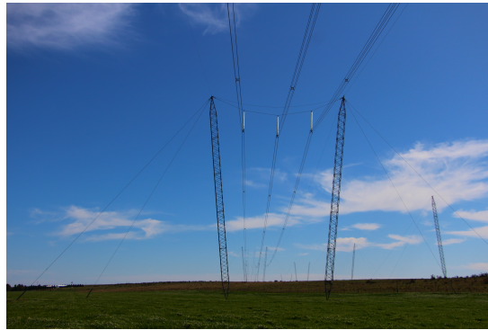
Figure 1: Photograph of an OTL with CR suspension towers.
